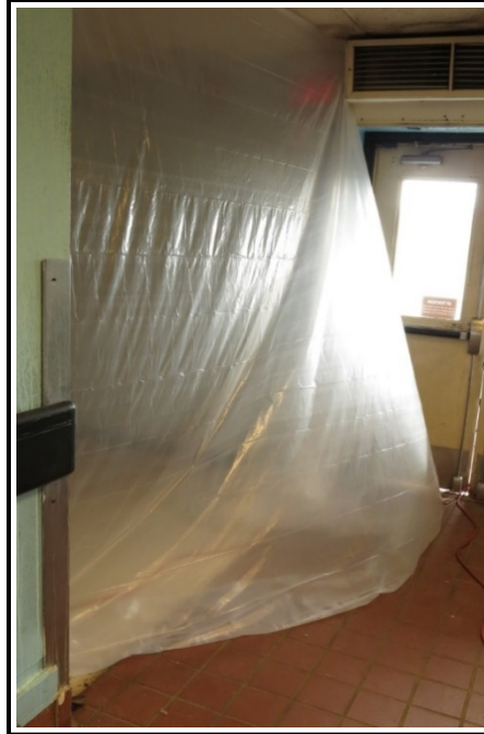
Figure 16. Positive pressure at various points within Bldg. 2261.
