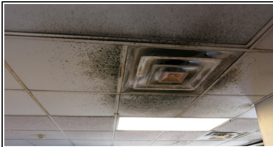
Figure 19. Mold growing near duct vents in Bldg. 2261.
